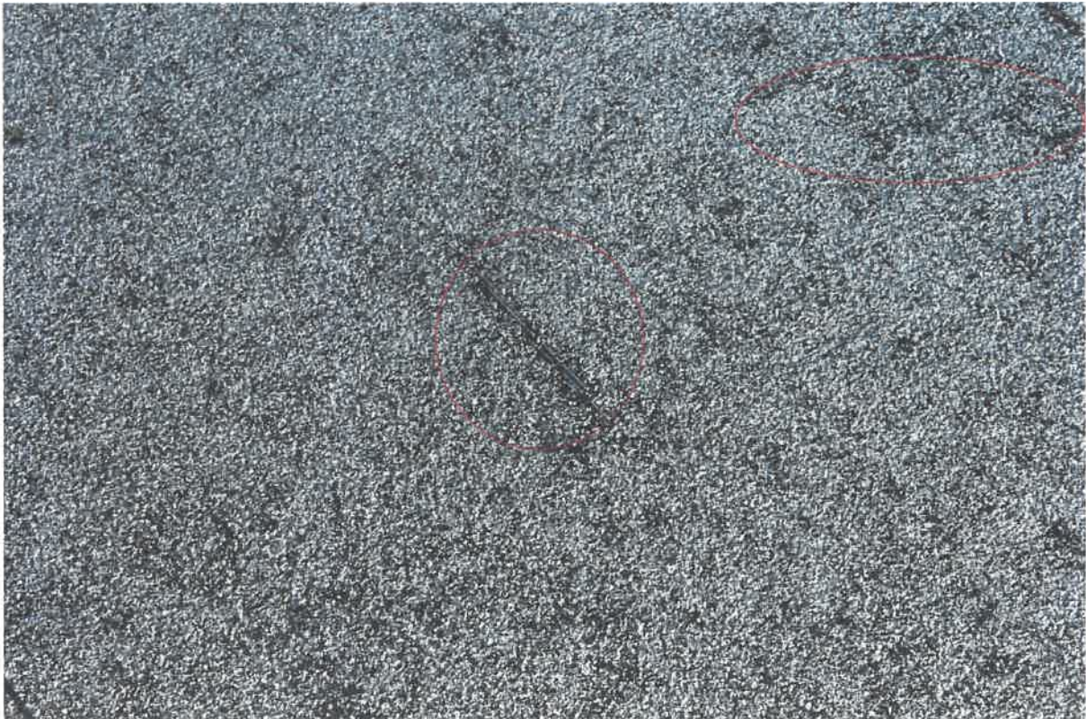
3.4 Detail of worn granular stone exposing fiberglass reinforcement.
