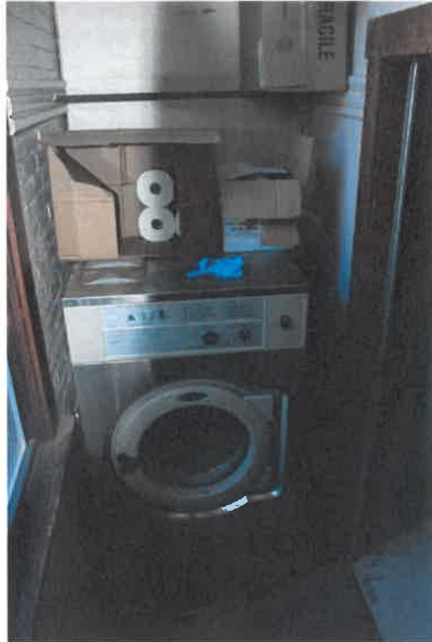
4.1 Washing machine in a means of egress stair
