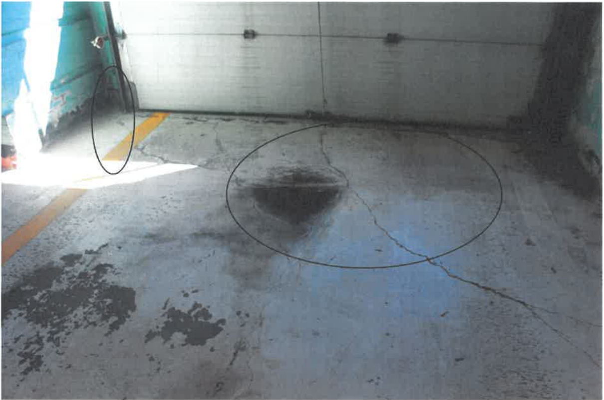
3.1 Bay 5 floor failure In corner failure radiates up brick wall
