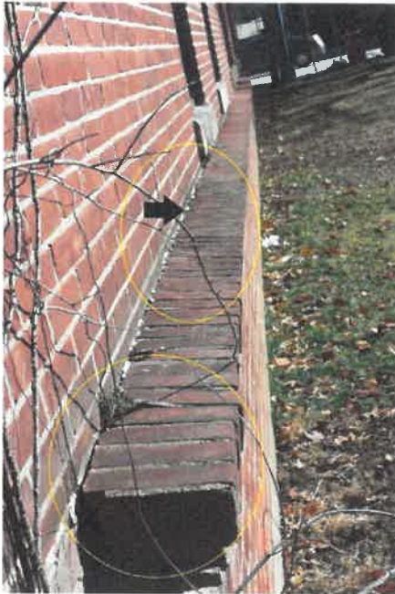
3.3 1960 Brick shelf improperly flashed and failing. Caulk joint (arrow) failed, but not a proper application
