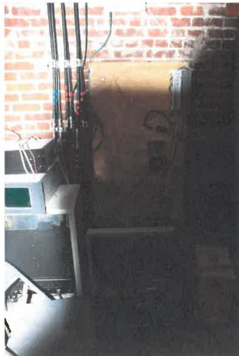
4.3 Communication equipment in upper tower attic. Concern is questionable roof pan has leaked and could affect equipment
