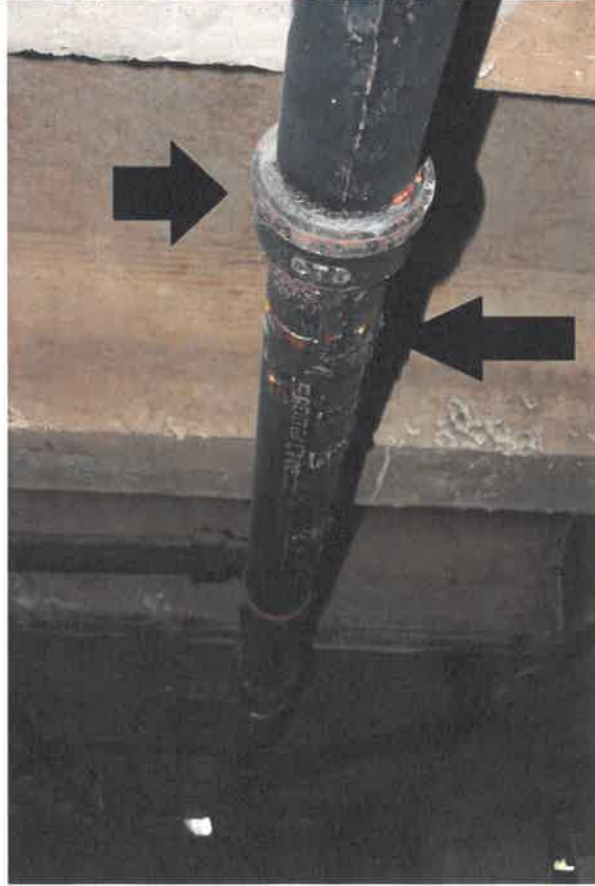
4.1 Leaking waste pipe joints and leaks in piping
