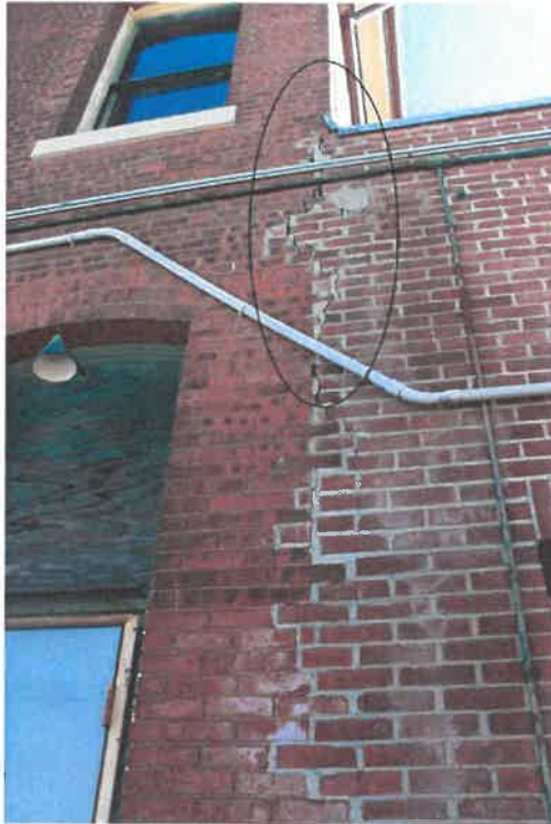
3.2 Significant brick movement main building at 1940s addition. Excessive water infiltration is occurring causing efflorescence and continual failure.
