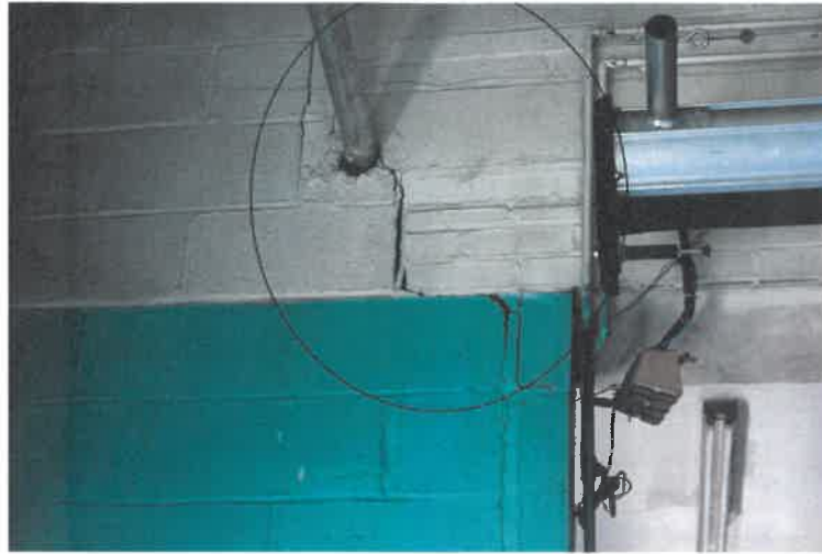
3.2 Interior wall of 1960 addition stress cracks at opening
