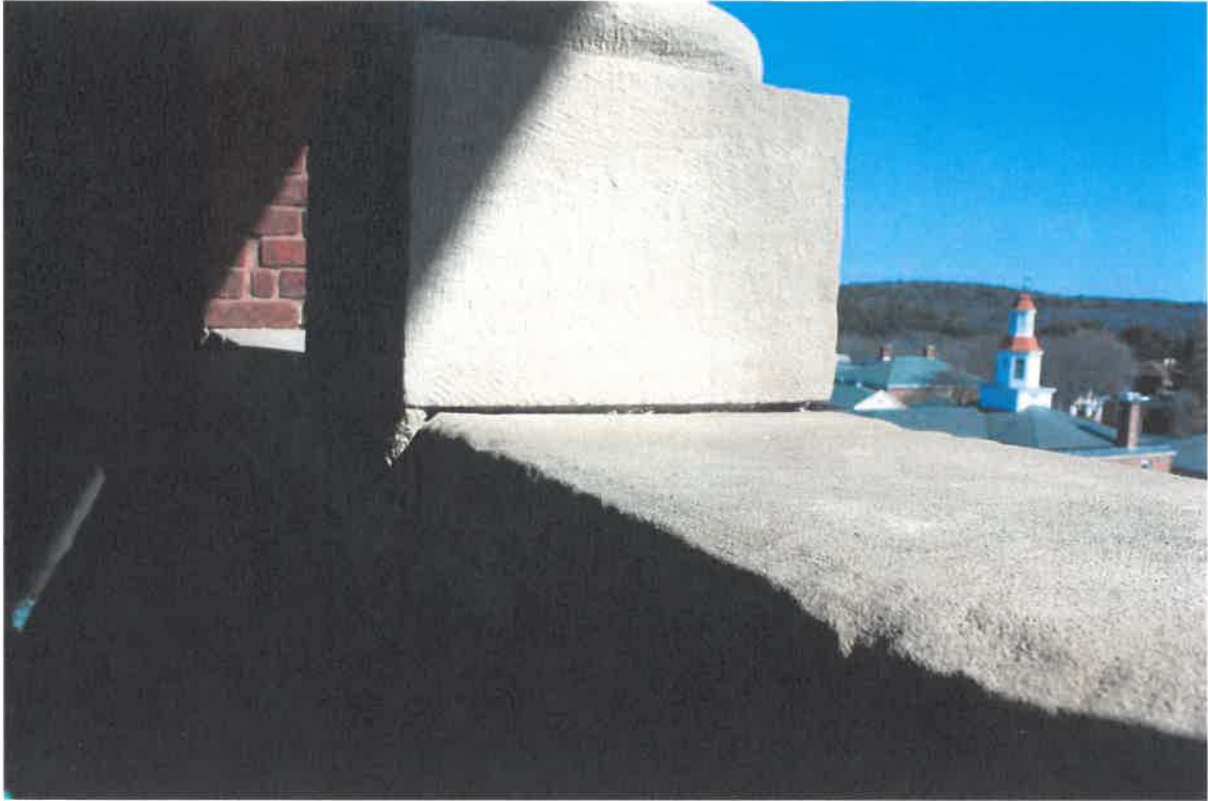
3.2 Tower column missing mortar
