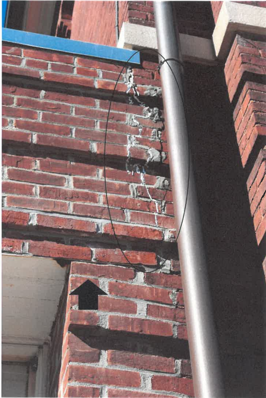
3.2 Significant brick movement and failure at front façade. Arrow shows rusting lintel that appears to have deflected and expanded opening mortar joint that has been filled with mortar.
