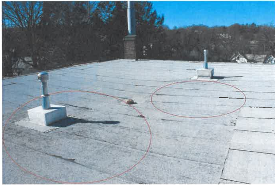
3.4 Apparatus bay roof. Roof granular stone facing is worn thin
