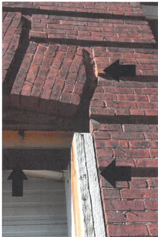
3.2 Added exposed lintel (rusting). Wood support not engineer to support masonry. Upper arrow indicates mortar joints opening up
