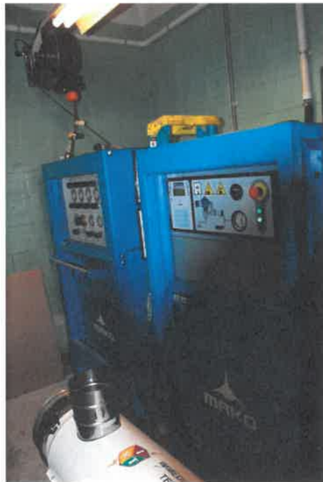
5.0 Scotts Pack filing machine located in the rear of the 1960 apparatus bay. No room separation as required per NFPA and Manufacturer.
