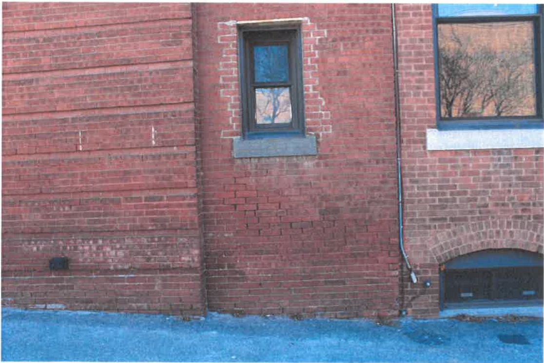
3.3 Typical areas of significant missing grout
