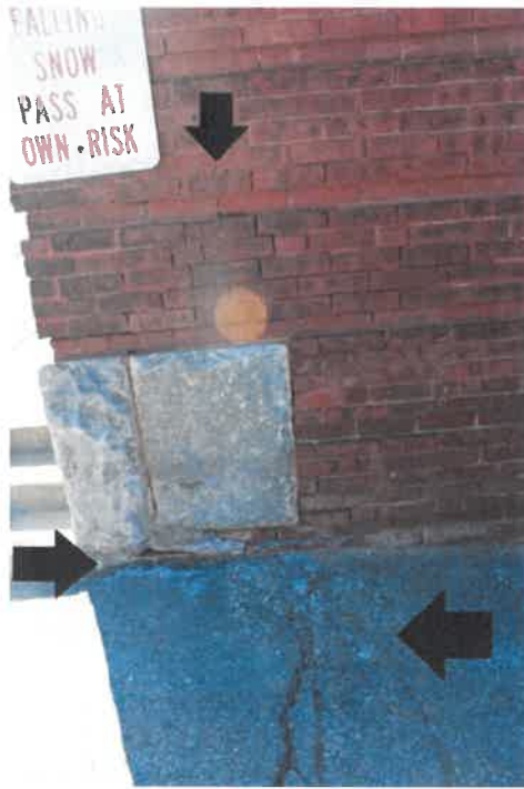
3.3 Typical mortar failure. Cornerstone stress cracking and poor mortar repairs
