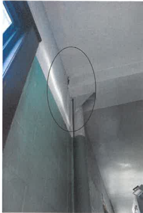
3.2 Interior beam at exterior addition wall pulling away from wall
