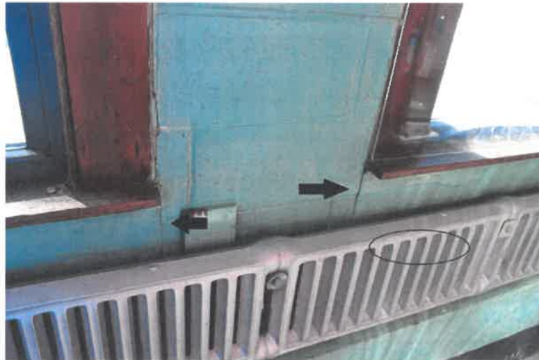
3.1 Bay 6 exterior wall stress crack through brick and block. Radiator is not in service
