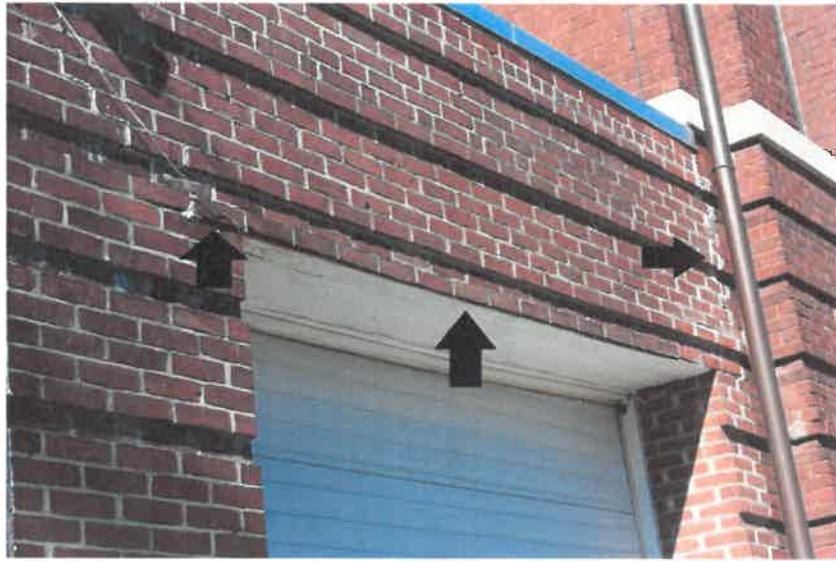
3.2 Bay 5 garage door lintel and mortar failure due to deflection, rusting and movement.
