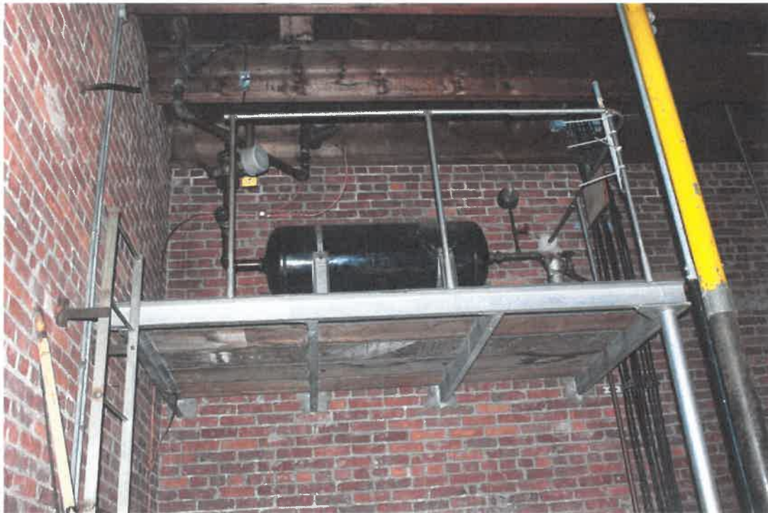
5.0 Bad air tank (air horn system) not in compliance or approved by State of Massachusetts.
