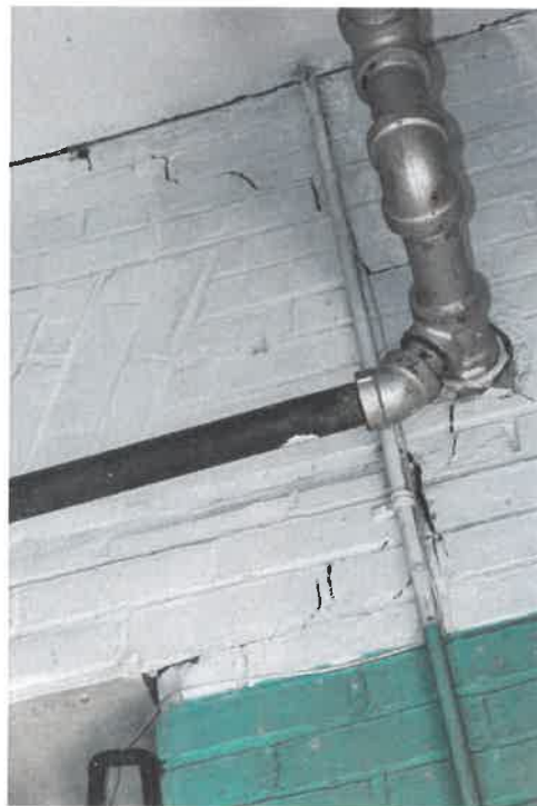
3.2 Addition building stress cracking of brick at interior wall
