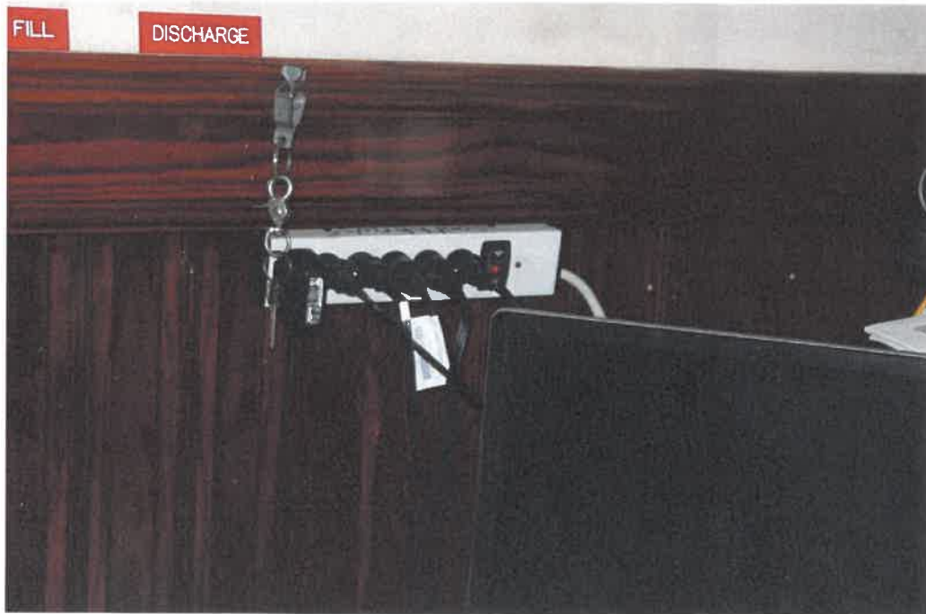
4.3 Typical electrical overloading of circuit due to lack of outlets.
