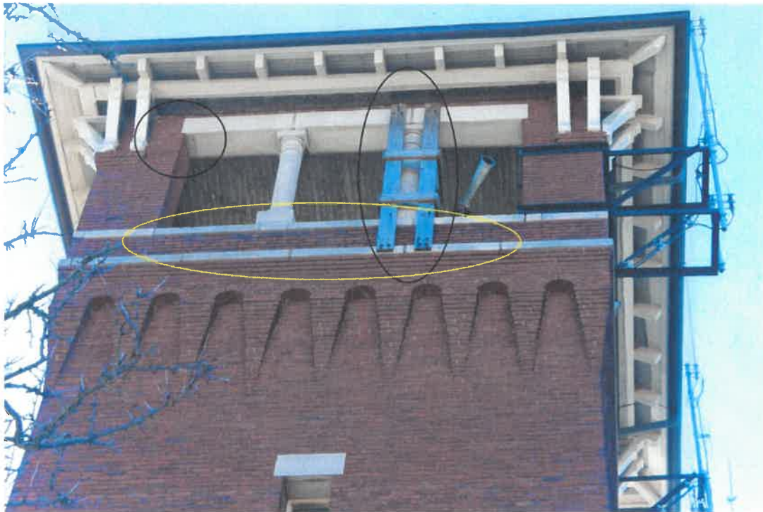
3.2 Wood Temporary support. Concrete lintel support area of concern. Brick and mortar damage (yellow) causing upper cast stone movement. Note: critical communications equipment on right
