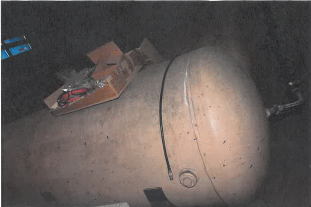
Operation air horn tank not in compliance with State of Massachusetts pressurized tank standards
