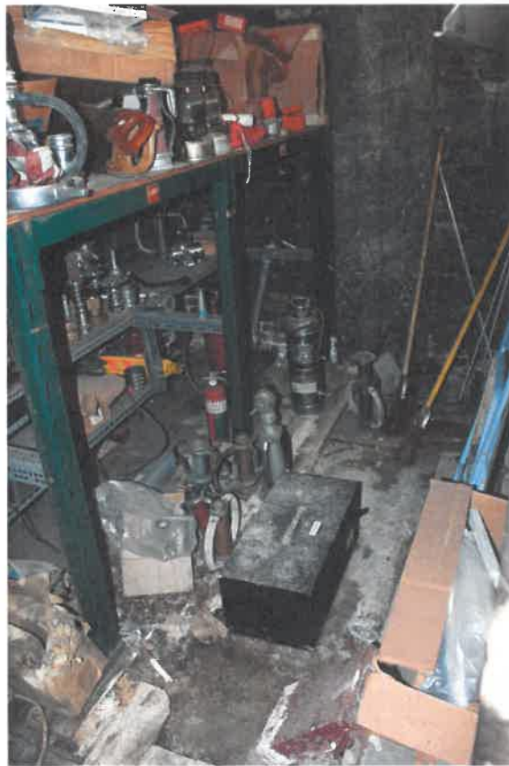
3.5 Basement storage affected by excessive moisture
